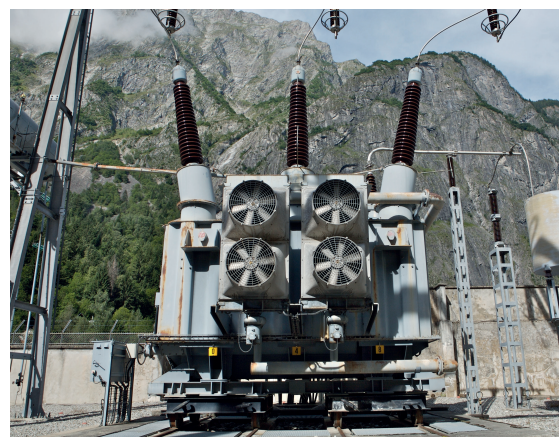
Plant output transformer
