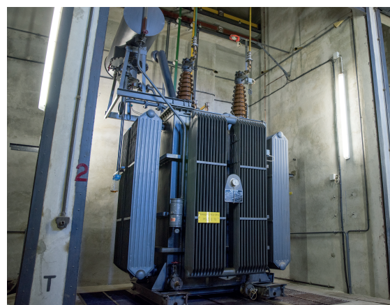
Transformer in the 63kV pumping station substation
